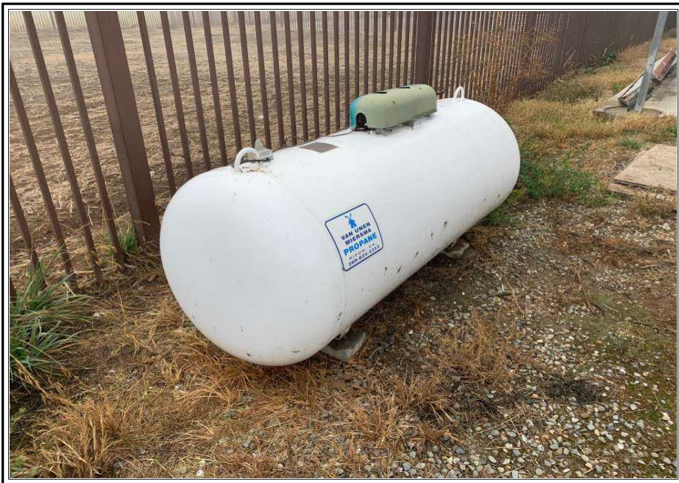
Propane tank for shop heating
