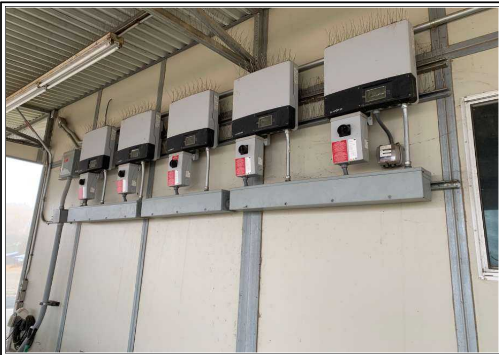
Solar inverter boxes for property
