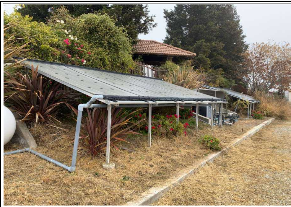
Passive solar heating for pool
