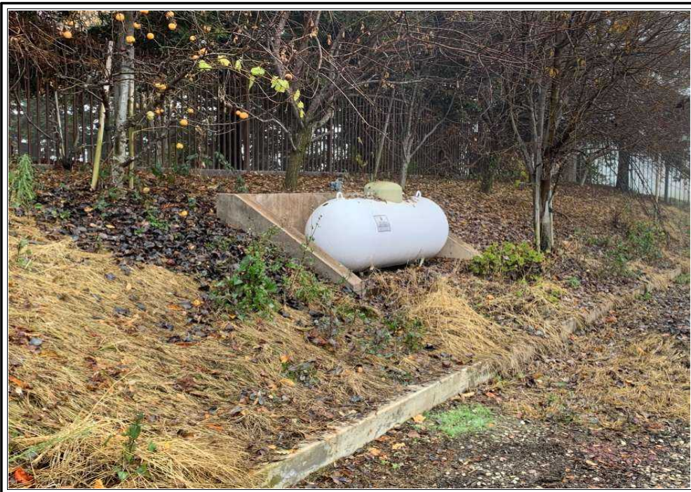
Propane tank for Accessory Unit
