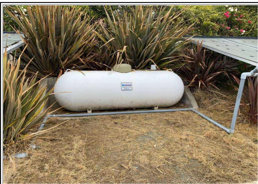
Propane tank for main dwelling
