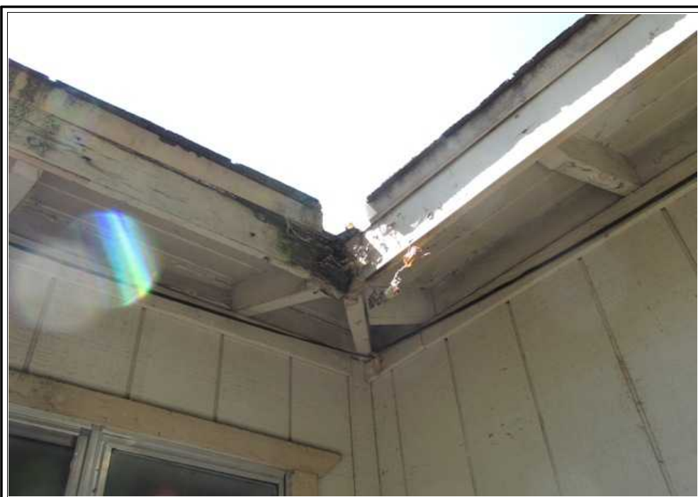
Area of damaged fascia board at rear of subject
