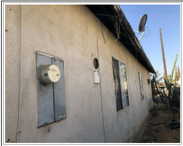
Exterior Side (Left Side) - Leaking water from composition roof. Roof and exterior trim is in need of repairs.
