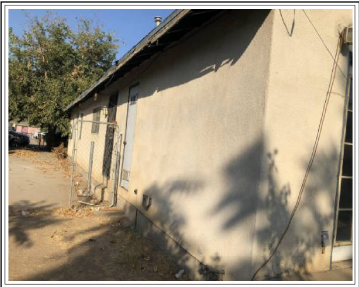
Exterior Side (Right Side) Roof and exterior trim is in need of repairs.
