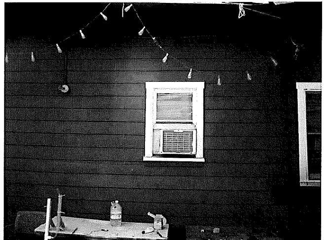
WINDOW AC UNIT
