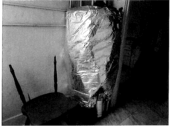
LAUNDRY HOOK-UPS-WATER HEATER
