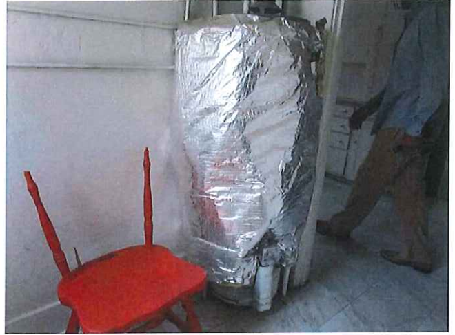
LAUNDRY HOOK-UPS~WATER HEATER
