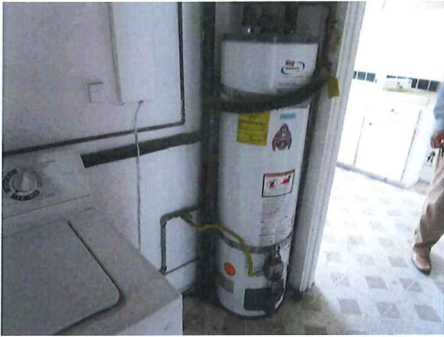
STRAPPED WATER HEATER
