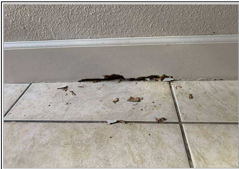
Signs of wood damage
