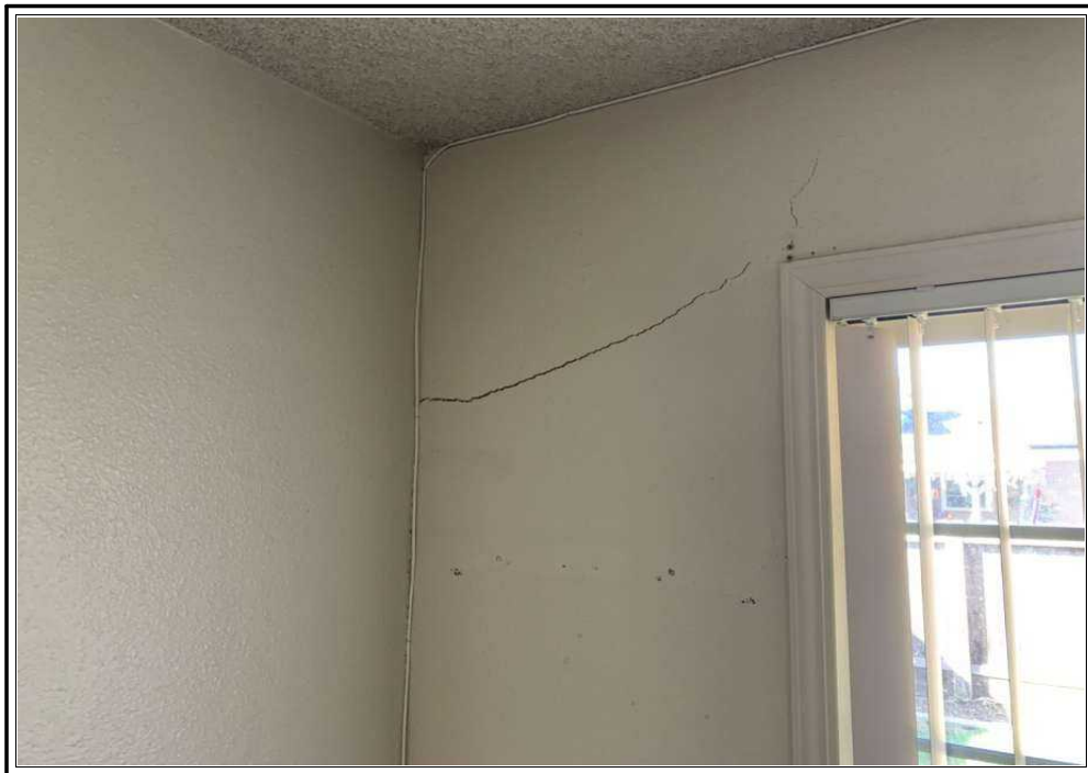
Drywall crack in master Bathroom
