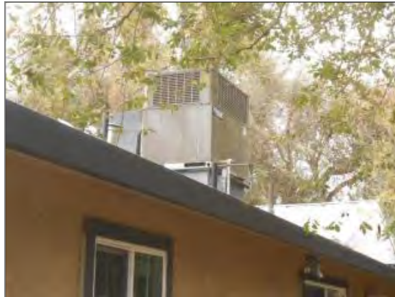
SFR – ROOF MOUNTED HVAC
