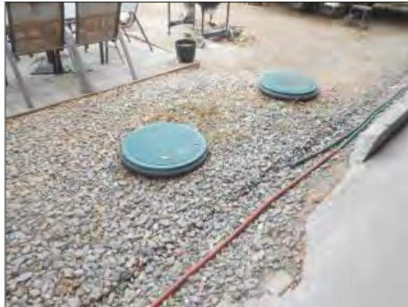
SEPTIC SYSTEM WEST OF COMMERCIAL BUILDING
