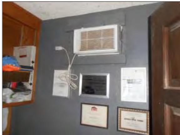
OFFICE AREA AIR CONDITIONER
