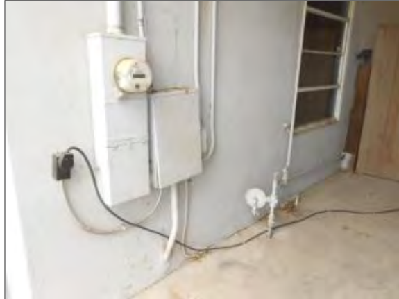
GAS & ELECTRIC UTILITY CONNECTIONS AT NW CORNER OF COMMERCIAL BUILDING
