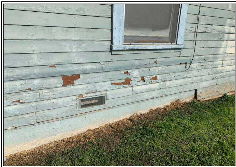
Exterior paint nearing end of effective life
