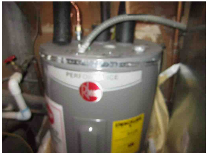
Braced H2O Tank
