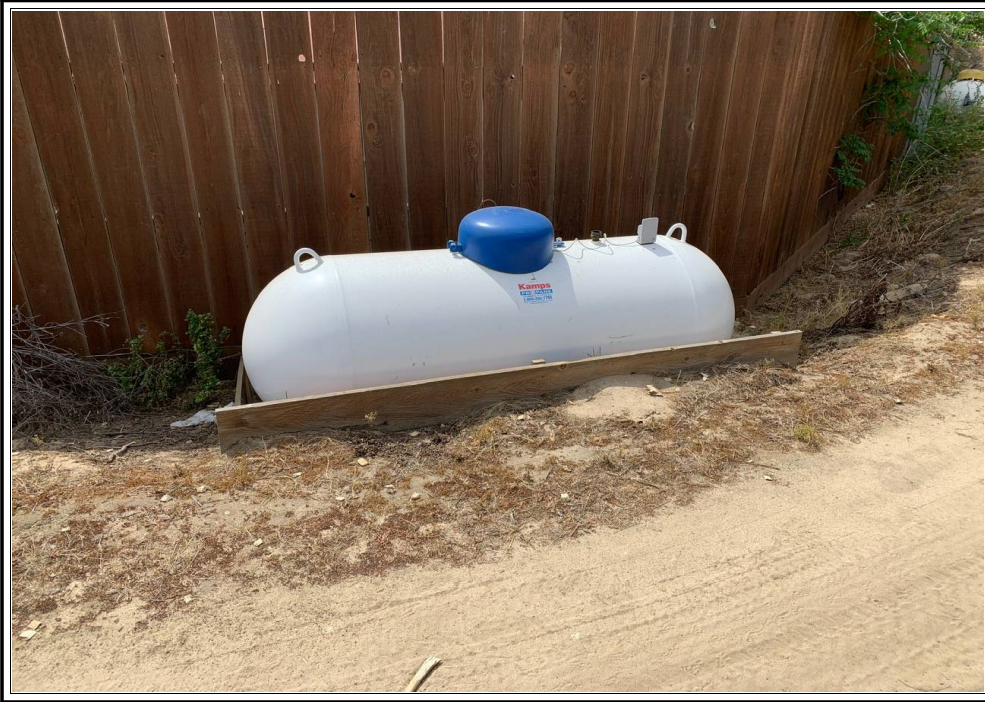
Propane tank for unit 14384
