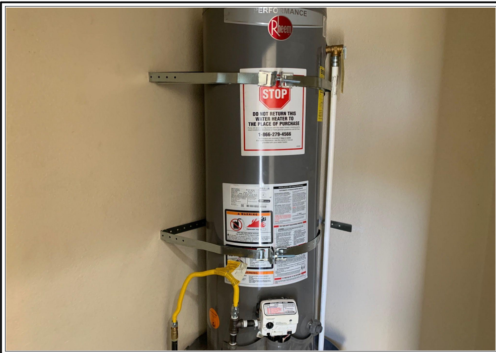
Double strapped water heater
