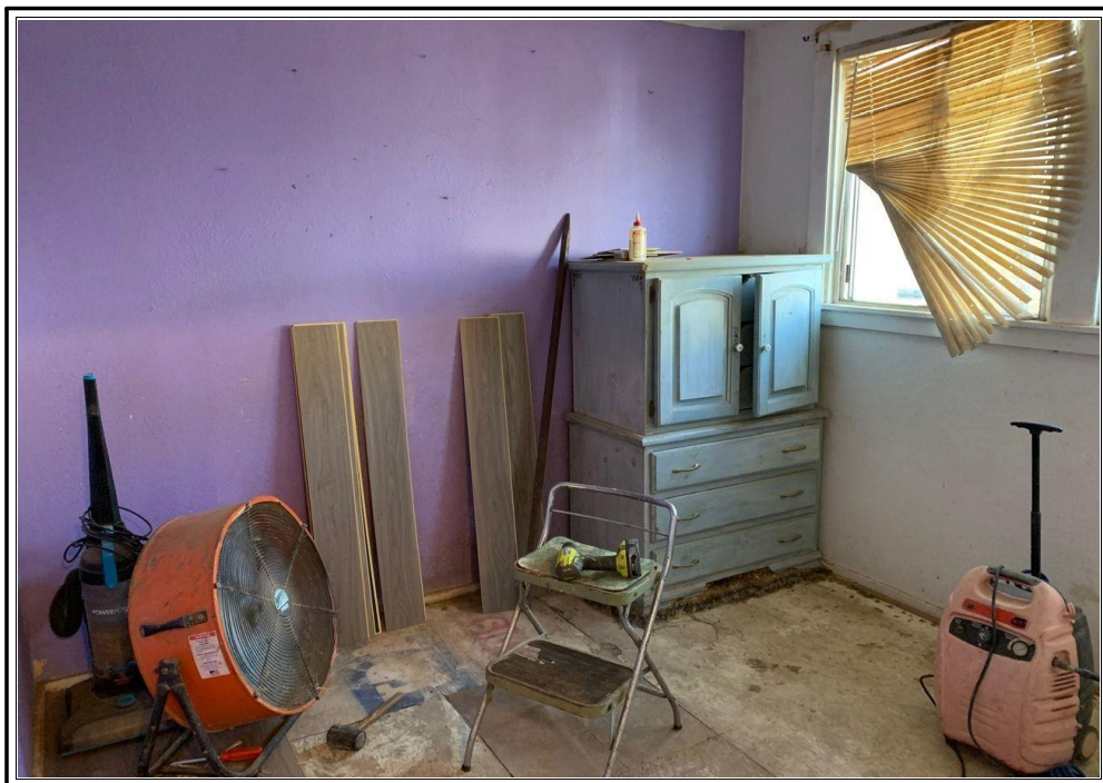
Bedroom - laminate flooring incomplete
