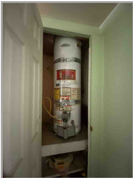
SUBJECT WATER HEATER
