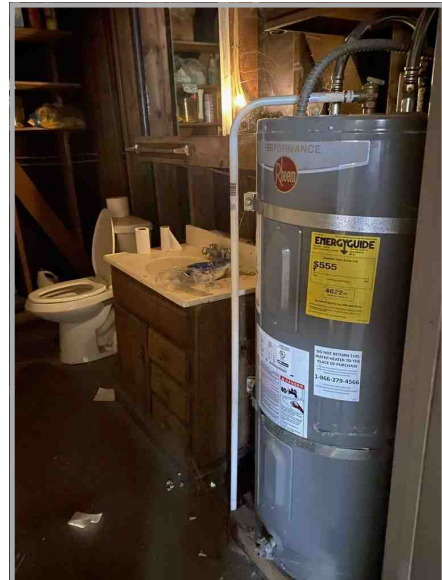
SUBJECT WATER HEATER 1/2 BATHROOM 1
