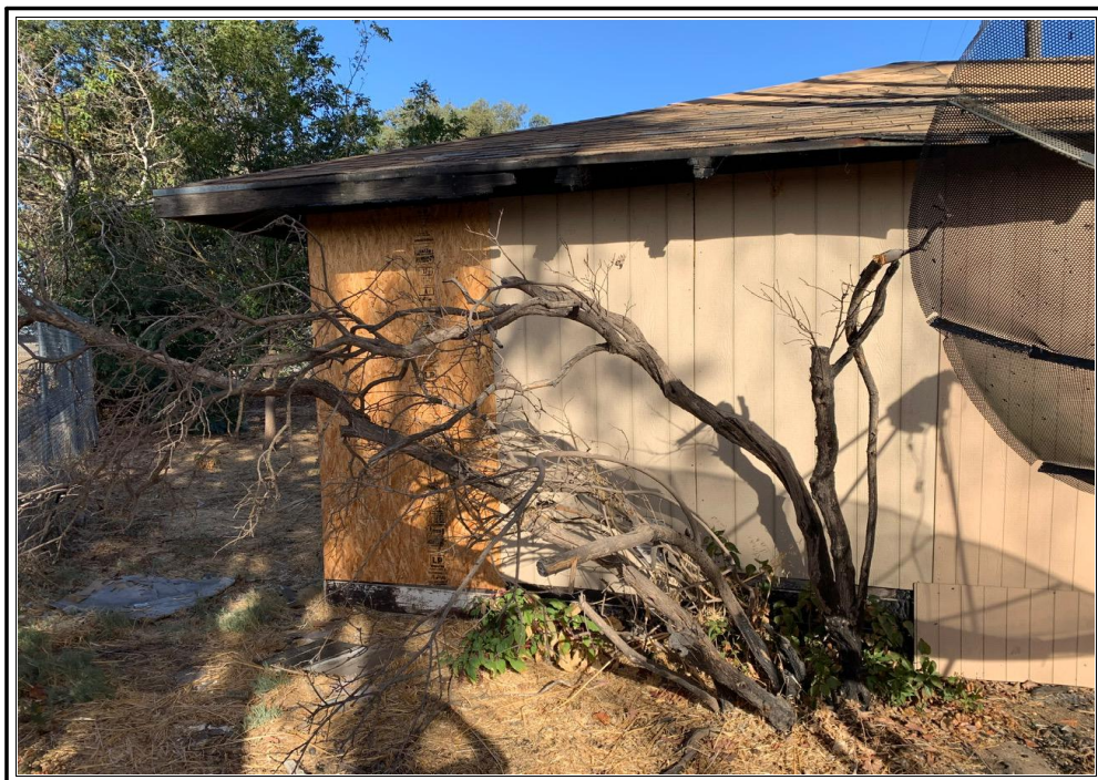
Side view of Garage showing exterior fire damage
