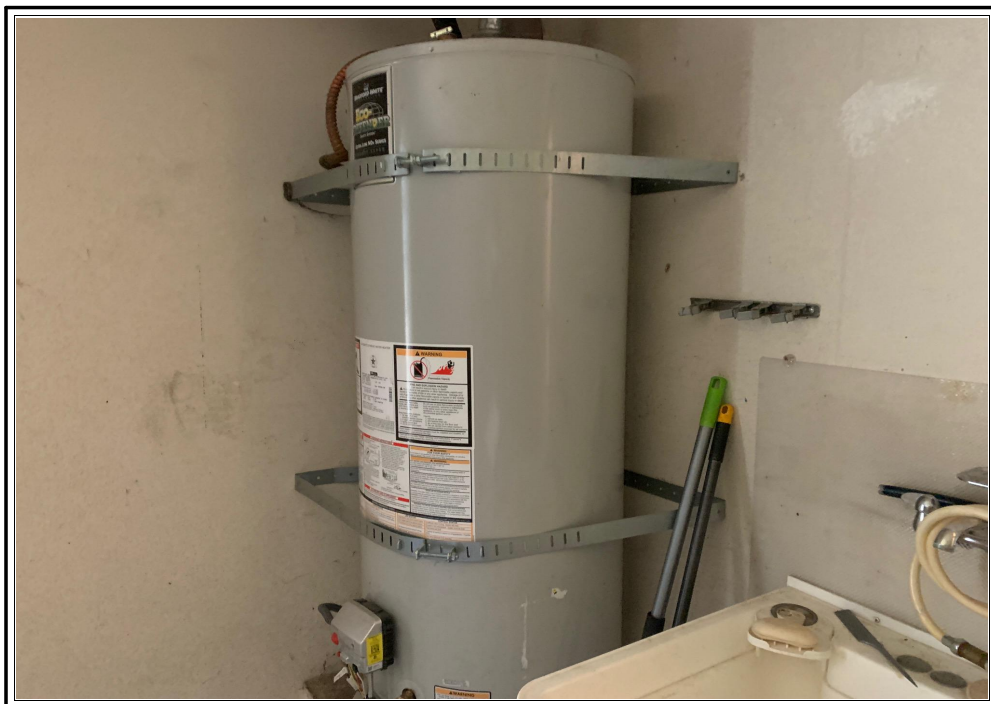
Double strapped water heater
