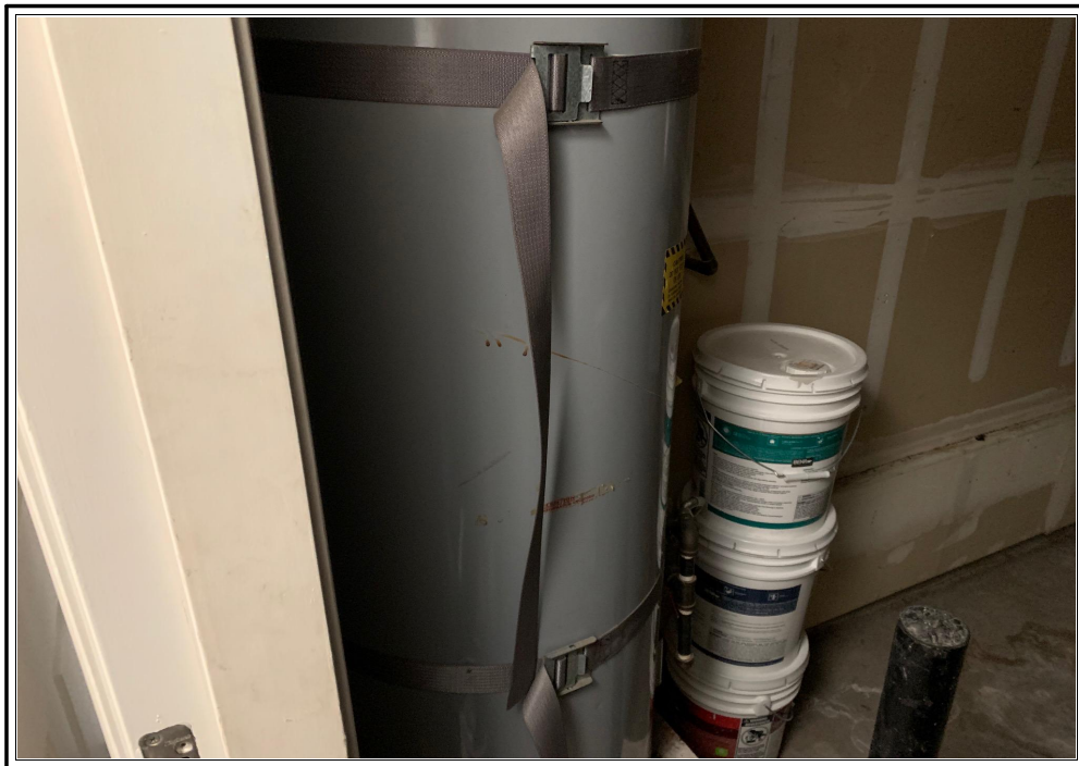
Double strapped water heater
