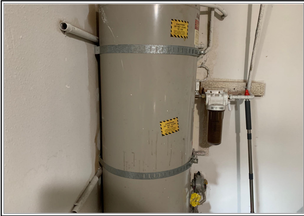
Double strapped water heater
