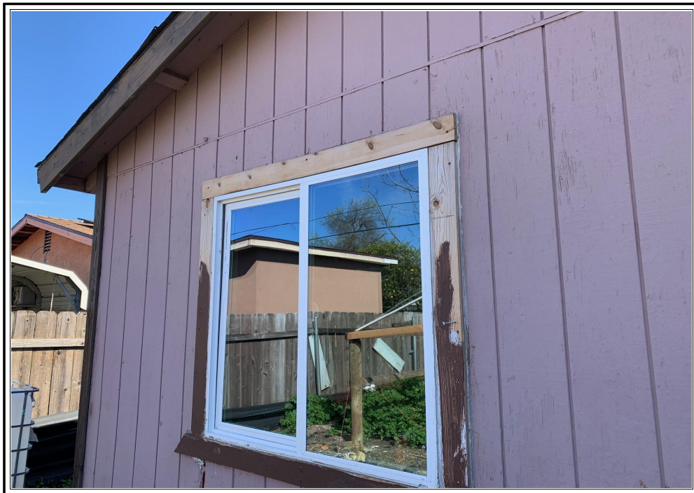
Window trim in need of painting
