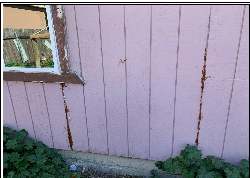
Rear siding in need of repair
