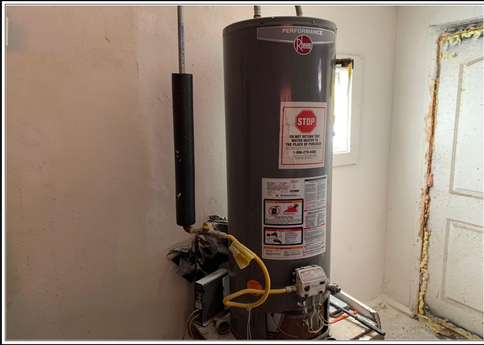
Water heater lacks straps and rear garage door has been sealed
