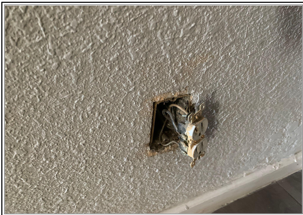
Outlet posing safety hazard
