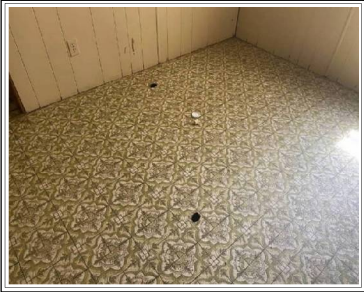
Floor damage in bedroom 3
