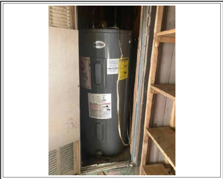
Water heater does not have straps Also does not appear to be operational
