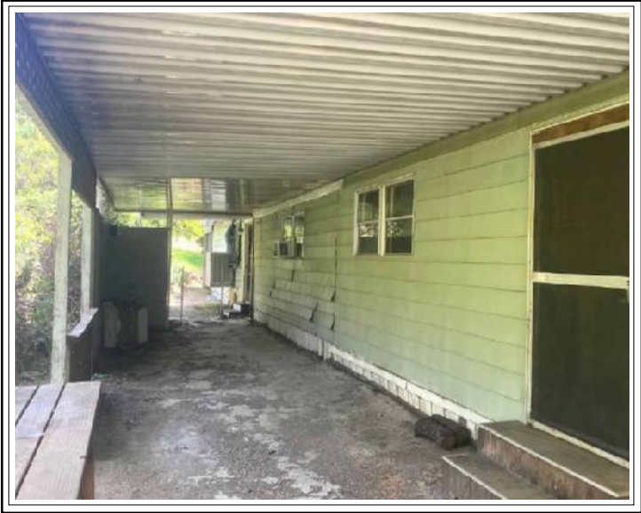
Covered Parking Siding Damage
