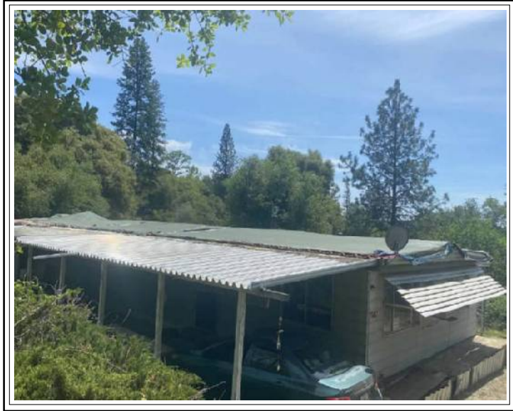
Roof has a tarp covering it Roof Damage
