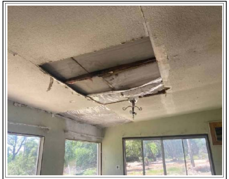
Ceiling Damage Bonus Room
