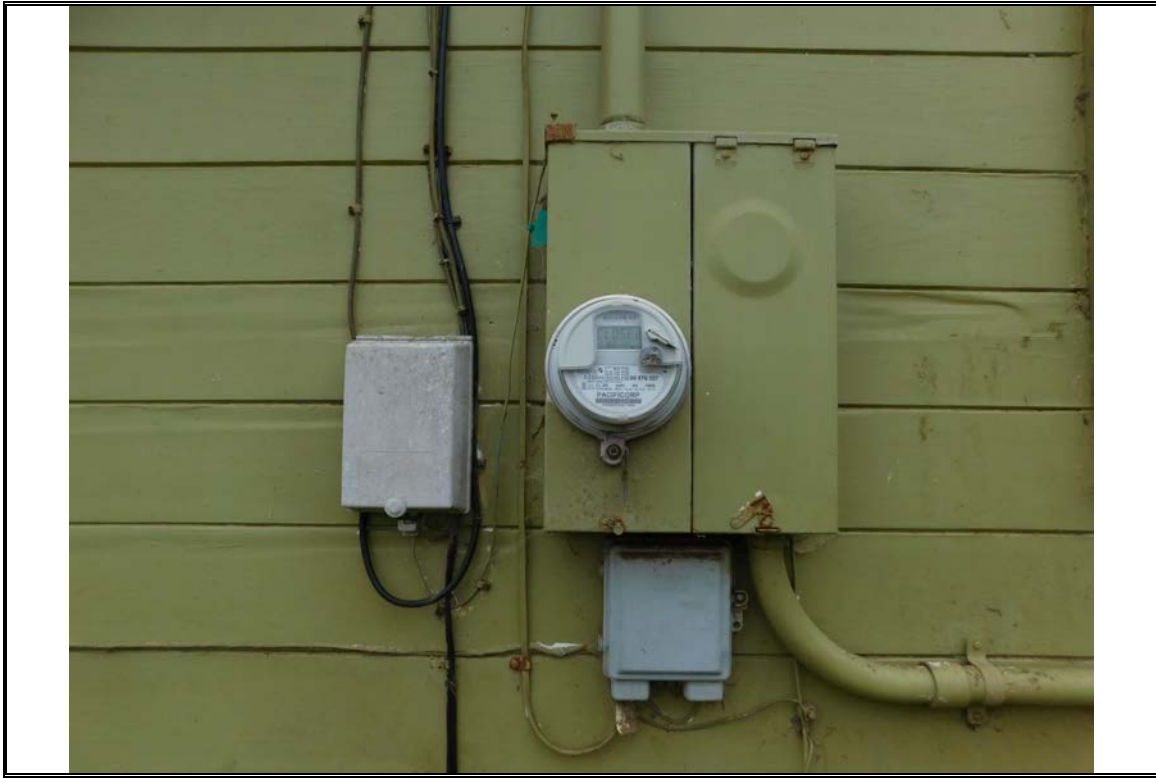
View of the subject 2/1 dwelling electrical service meter
