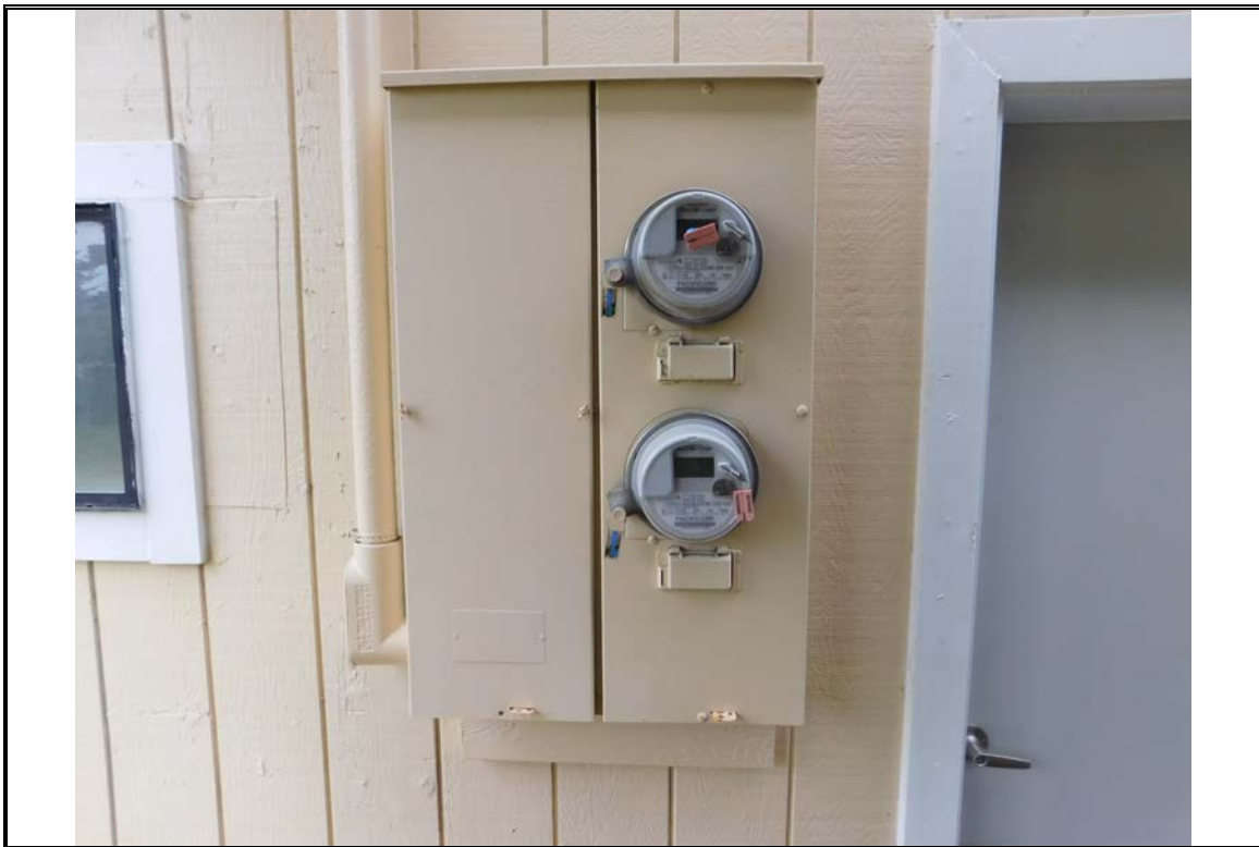
View of the two subject office electrical service meters
