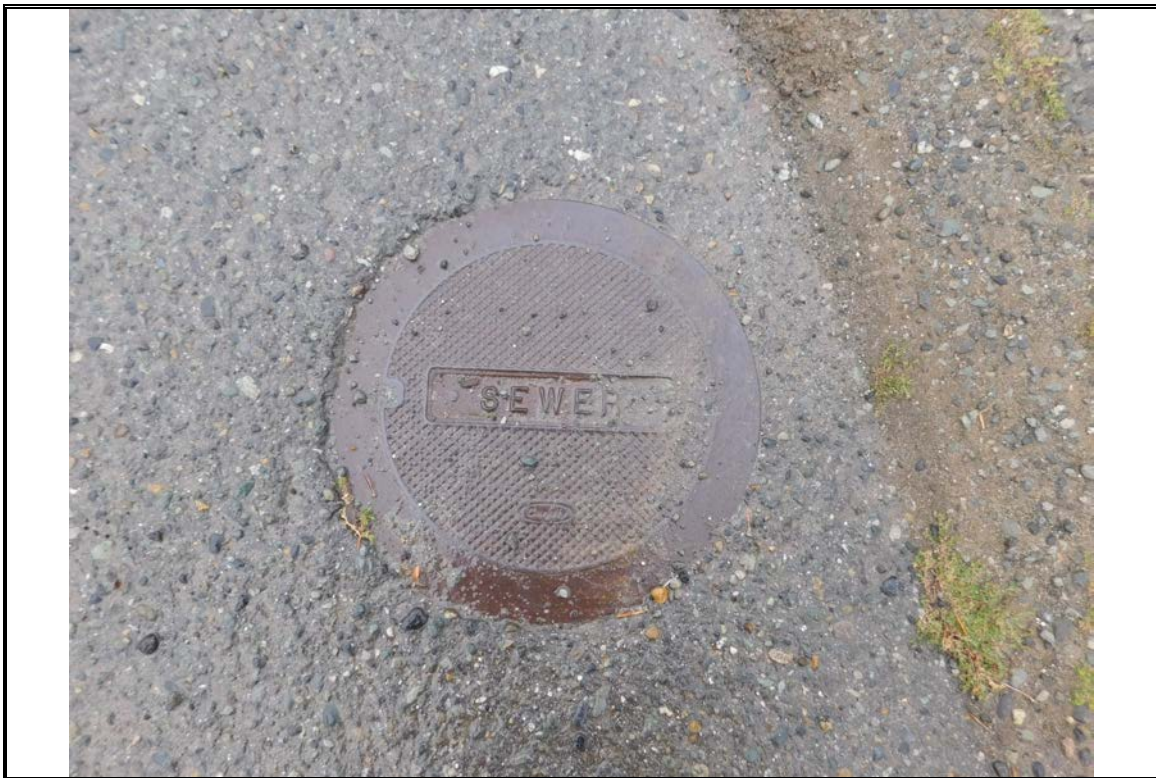
View of the subject sanitary sewer cover near the subject Northcrest Drive frontage
