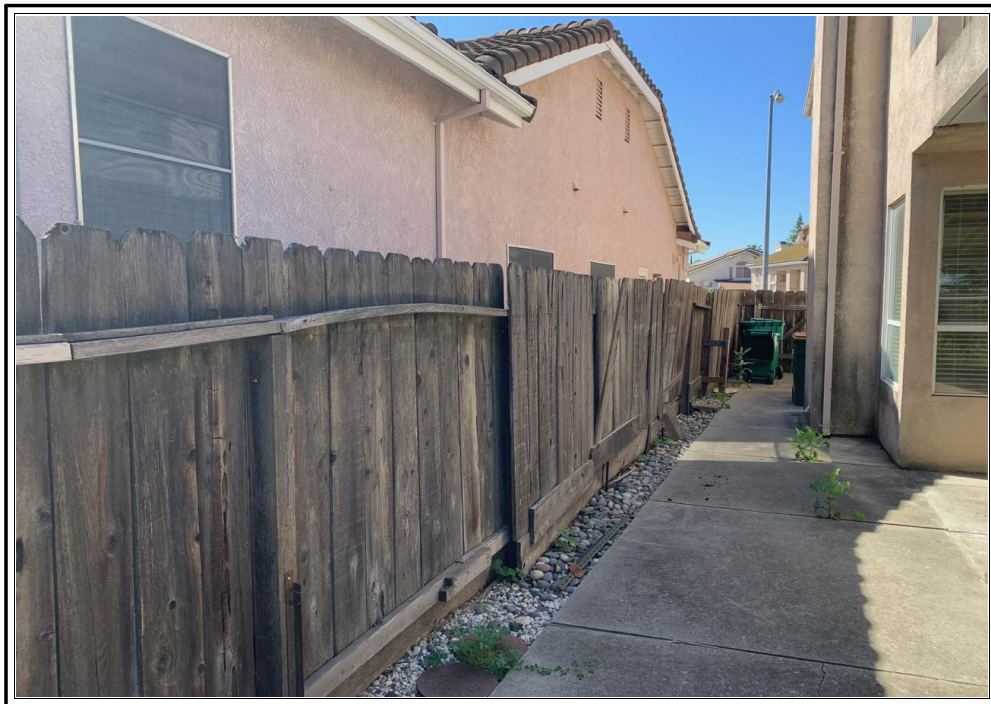
Side fencing in need of repair
