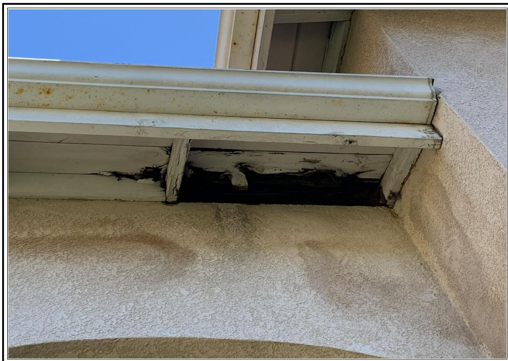
Wood damage to eaves
