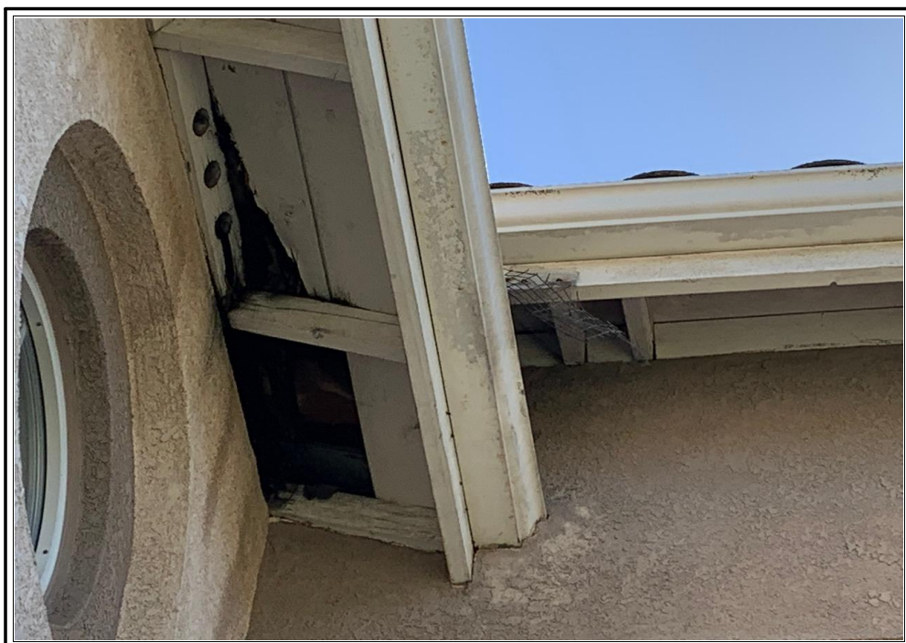
Wood damage to eaves
