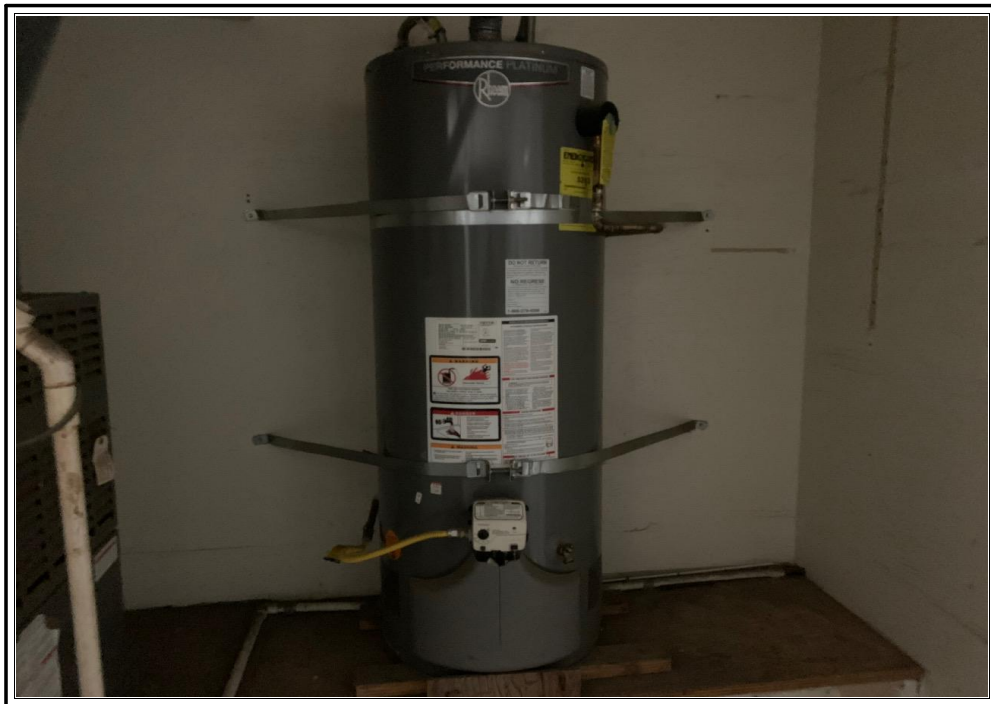
Double strapped water heater
