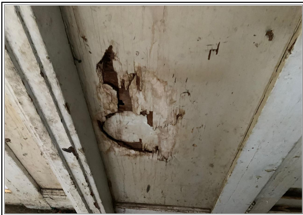
Damage to interior wall
