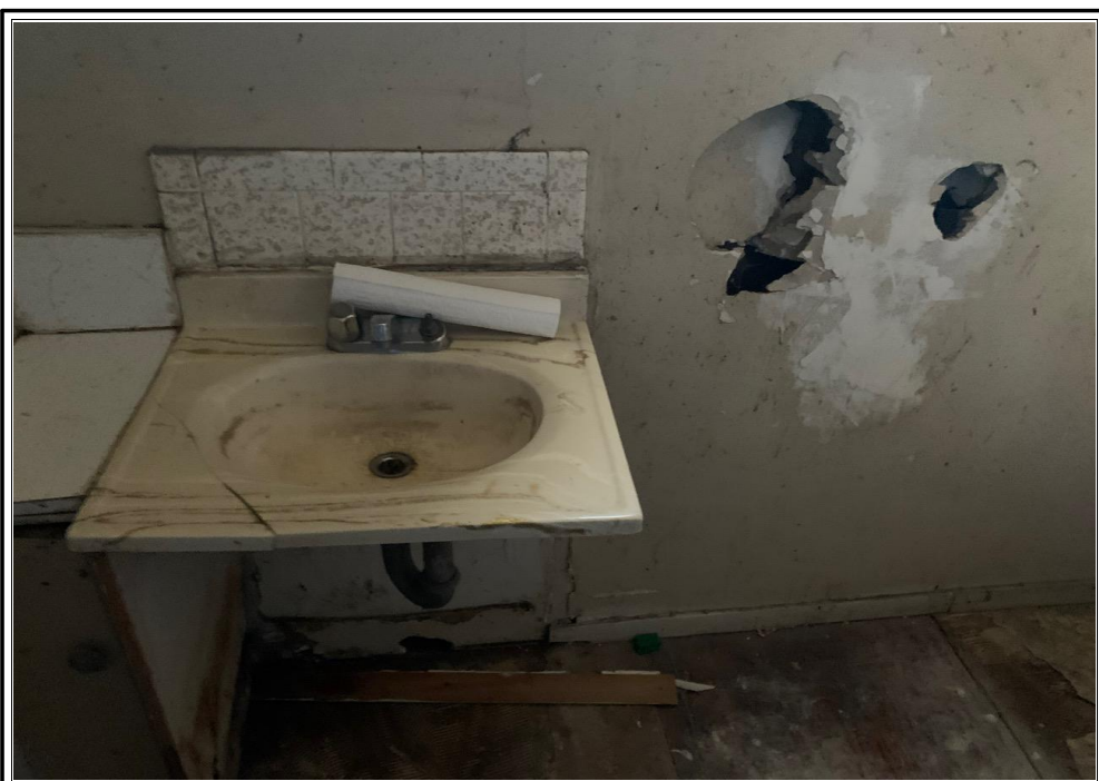
Additional view of Bathroom showing damaged to wall
