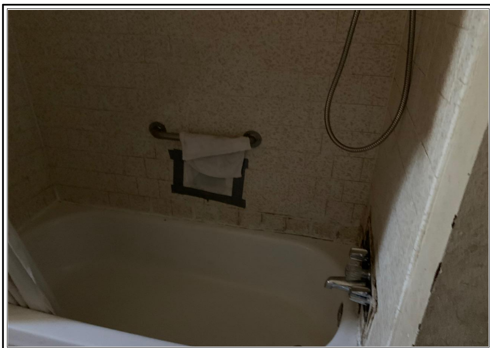
Damaged tile in tub/shower
