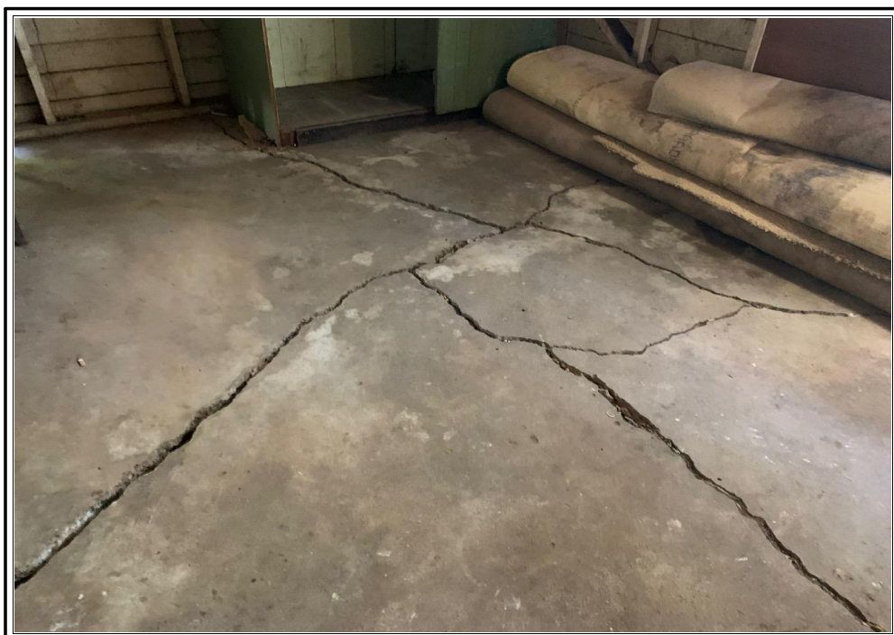
significant cracking to foundation in Porch/Laundry area
