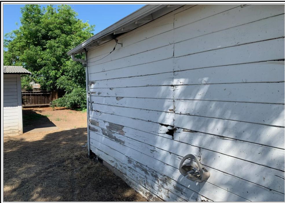
Damaged exterior siding and paint at end of physical life
