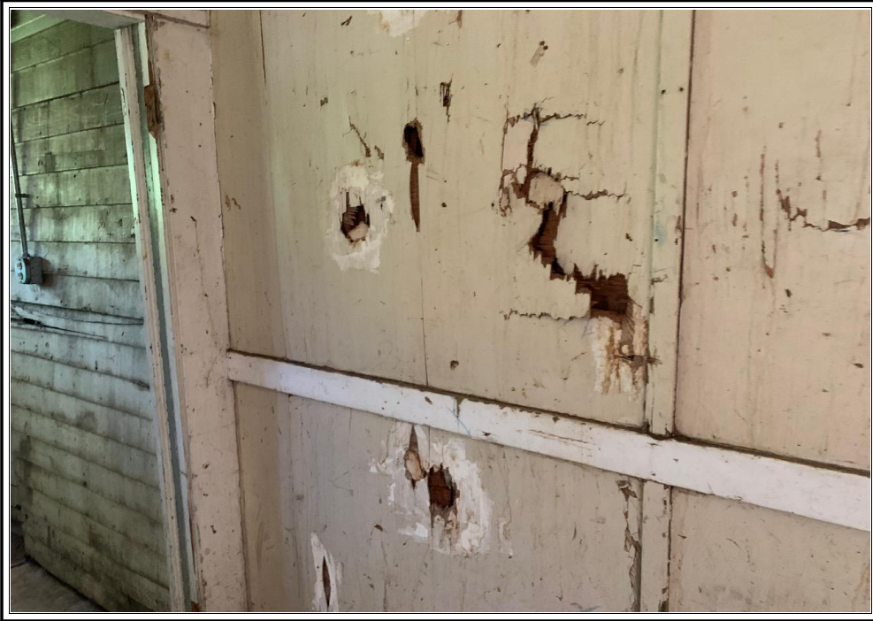
Damaged interior walls
