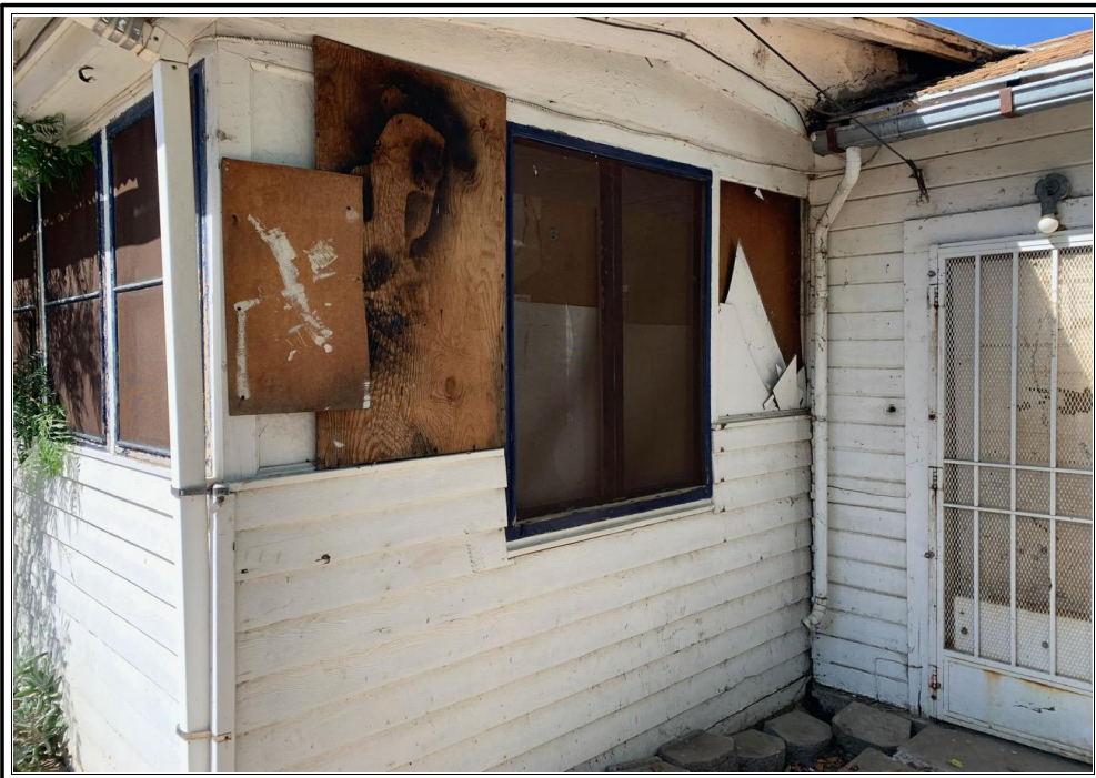
Boarded and broken windows
