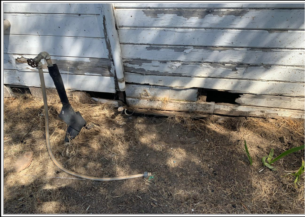
Damaged exterior siding
