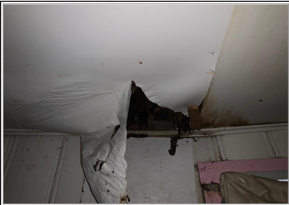
Ceiling damage in Bedroom
