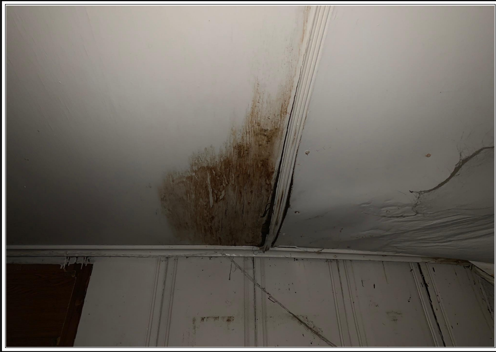
Ceiling damage in Bedroom
