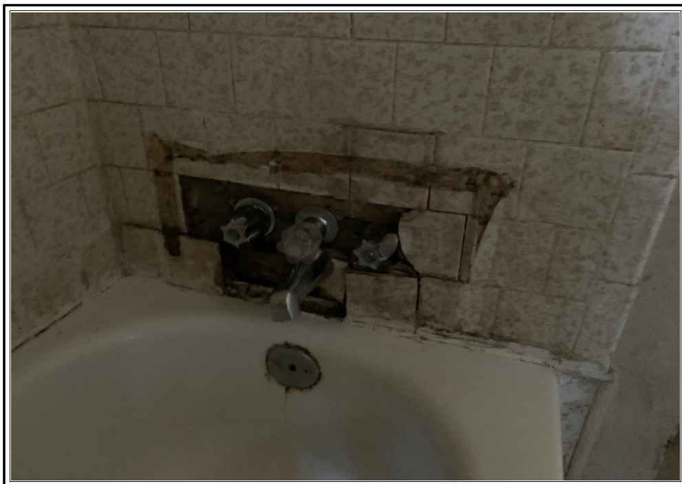
Damaged tile in tub/shower
