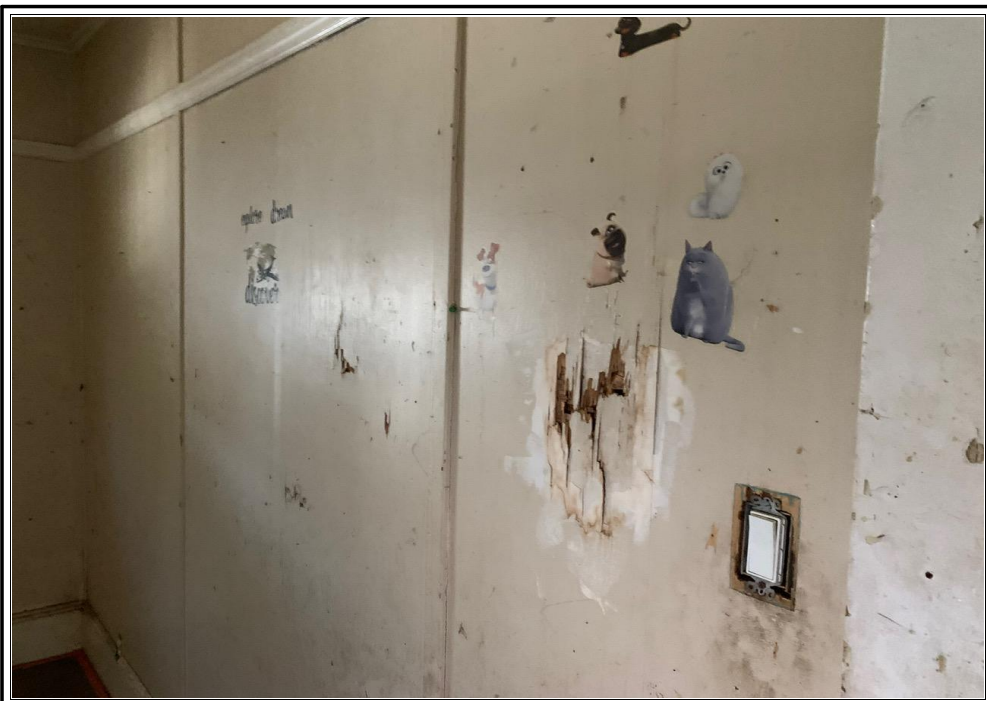
Damaged interior walls
