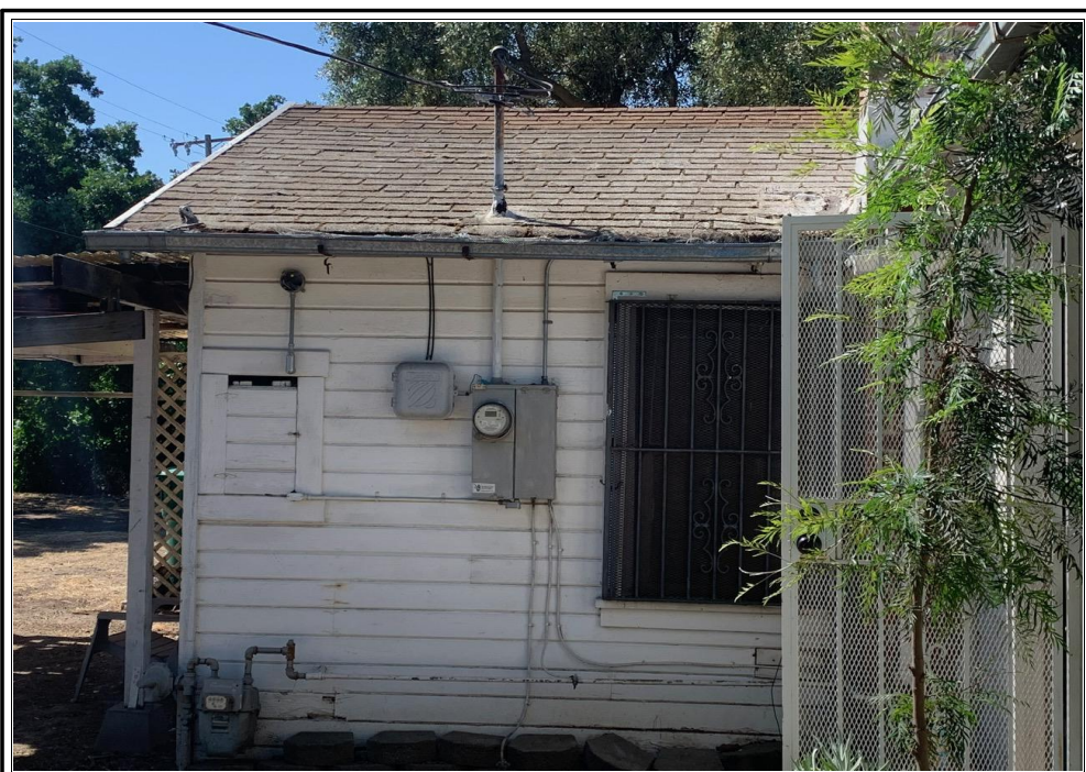
View showing poor condition of roof
