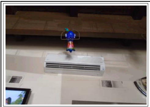
Wall Mount A/C Unit in Dining Area/ Restaurant
