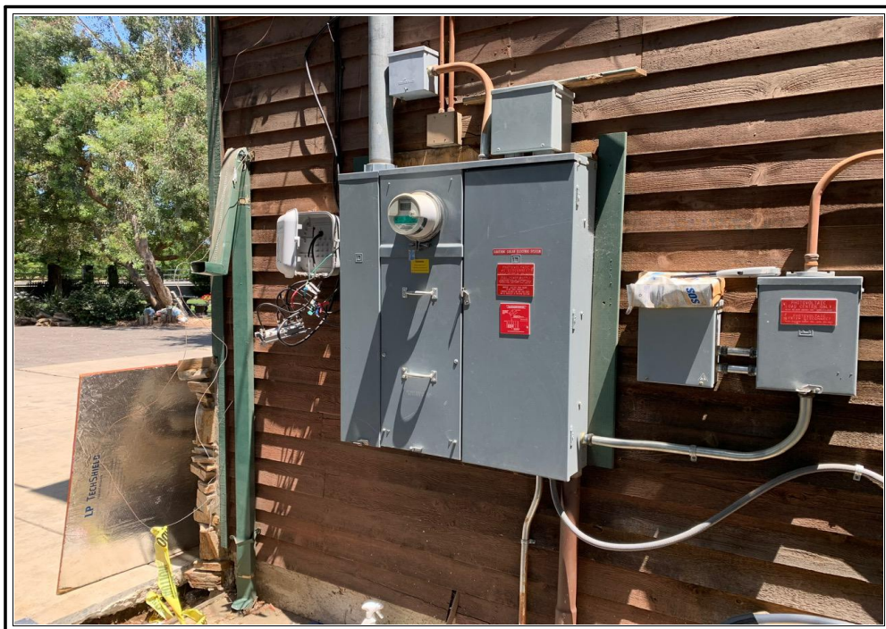
Solar PV system - Owned
