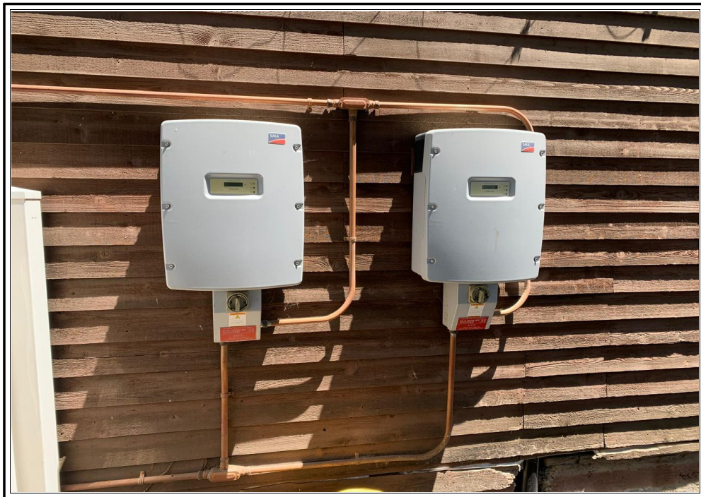
Solar PV system - Owned
