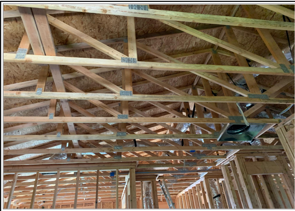
Interior view of Accessory Dwelling HVAC ducting installed
